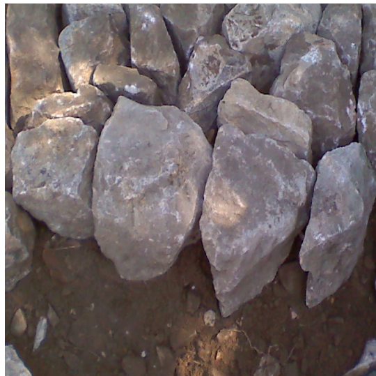
A close-up of the paving being replaced; again, no mortar.
